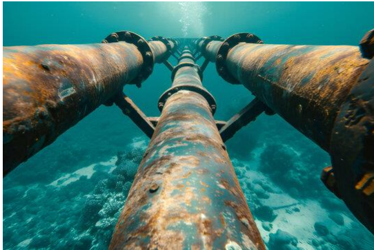
Figure 1: rusting of pipelines in the sea
